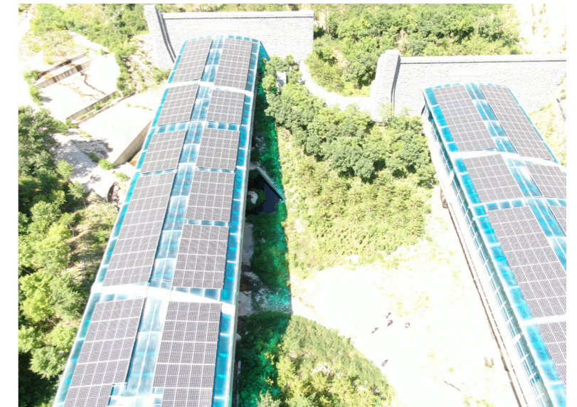
Rooftop Solar Panels of Beijing-Chongli Expressway Zhangshanying
