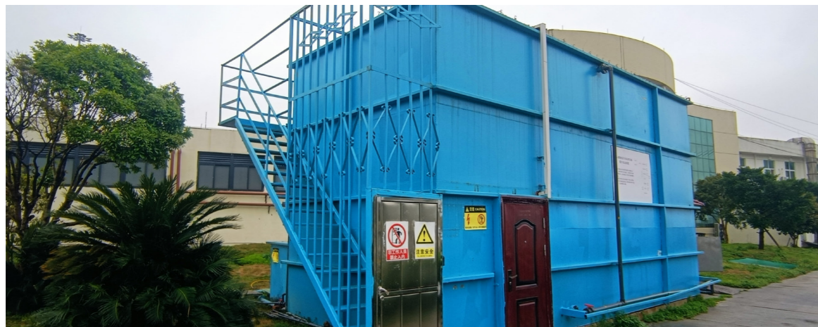
Qingjiang Service Area Sewage Treatment Station
