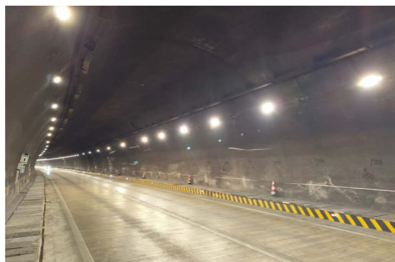
CMCR Cenxing and Cenwu Expressways tunnel lighting
